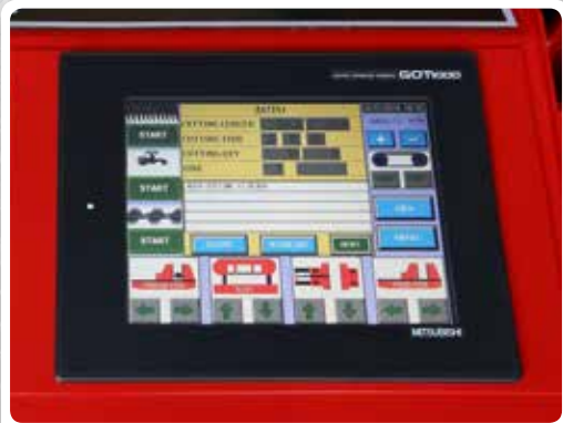
PLC Control Panel - Inverter
