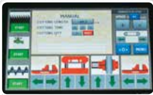
Inverter - PLC Control Panel
